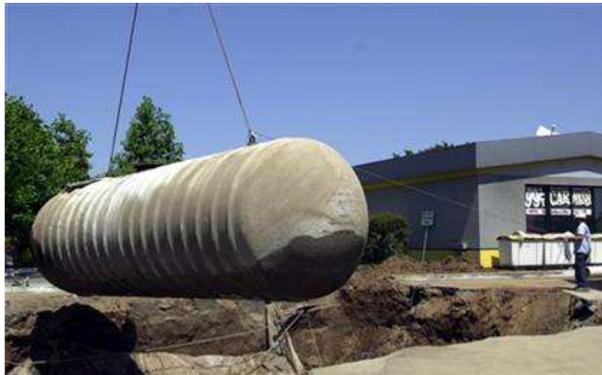
Figure (2). A damaged underground fuel tank in California, USA. [3]
